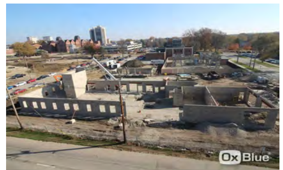
Installed video camera for time lapse photography to capture and archive construction.
