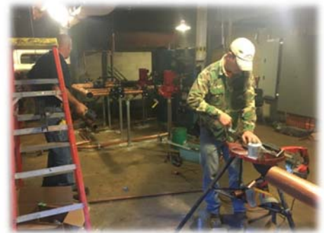
Community Activity Center Boiler
